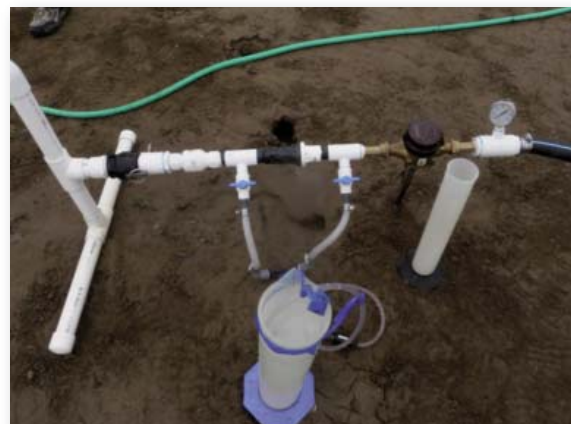
Figure 3: Mazzei injector setup with inline flow meter.
