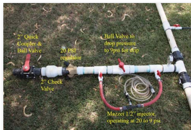
Figure 2: Mazzei injector and line setup.
